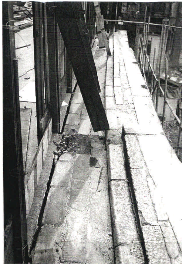
Plate D6.11 - Retaining Wall at Circular Pathway - Detail of the Cracks on the Pathway (I)
