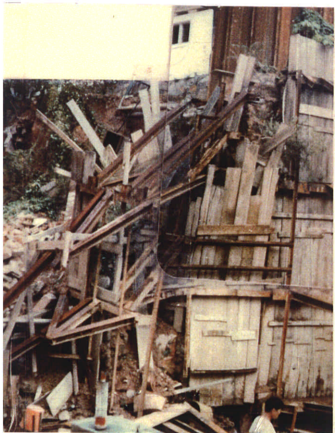
Plate D8.7 - Retaining Wall at Fat Hing Street - Enlarged View of the Collapsed Wall and the Deflected Shoring Adjacent
