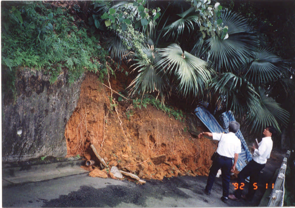
Negative No. I9221614 Taken on : 11-5-92 Description : Failure of a soil cut slope affecting a private access.
