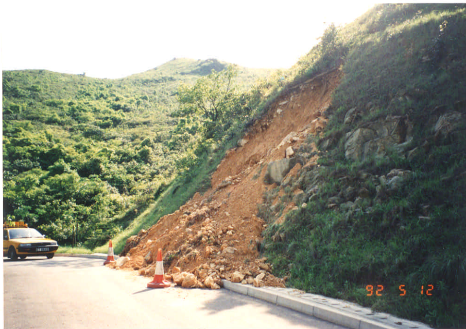
Negative No. MW9211519 Taken on : 12-5-92 Description : Failure of a soil cut slope resulting in the partial blockage of a road.
