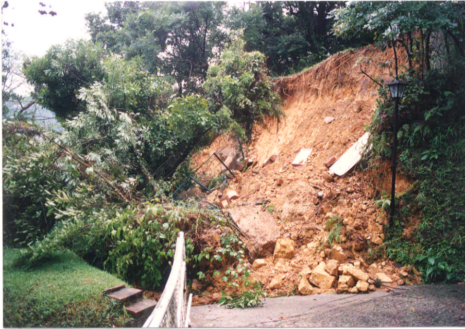
Negative No. I9220814 Taken on : 9-5-92 Description : Failure of a soil cut slope resulting in the blockage of a private access.
