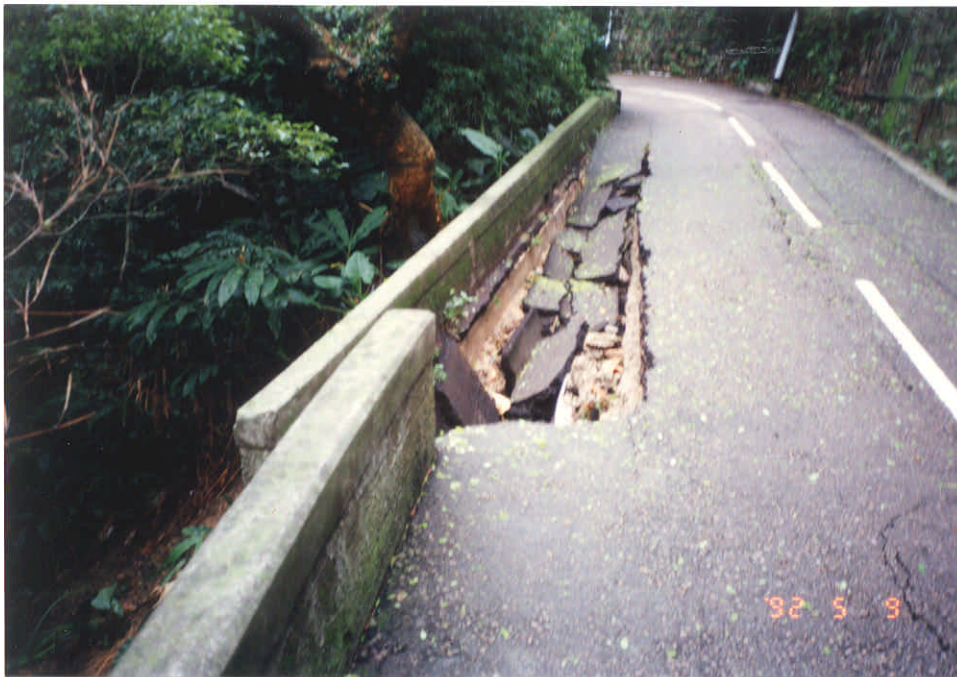
Negative No. A9206704 Taken on : 9-5-92 Description : Major failure of a retaining wall resulting in ground subsidence and the closure of two road lanes.
