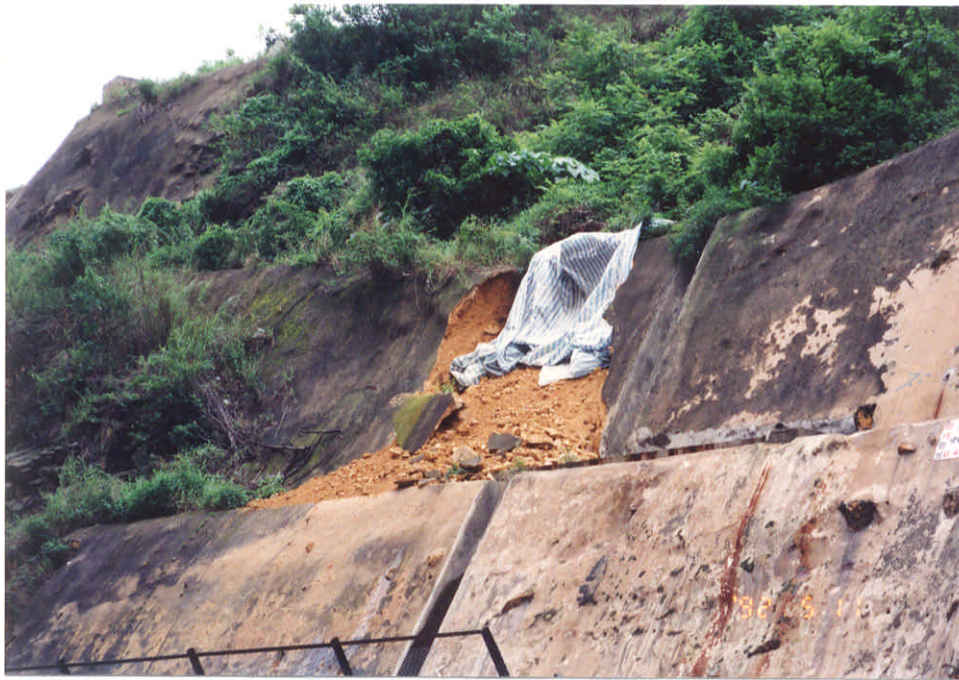
Negative No. MW9210806 Taken on : 11-5-92 Description : Failure of a soil cut slope affecting a pedestrian pavement.
