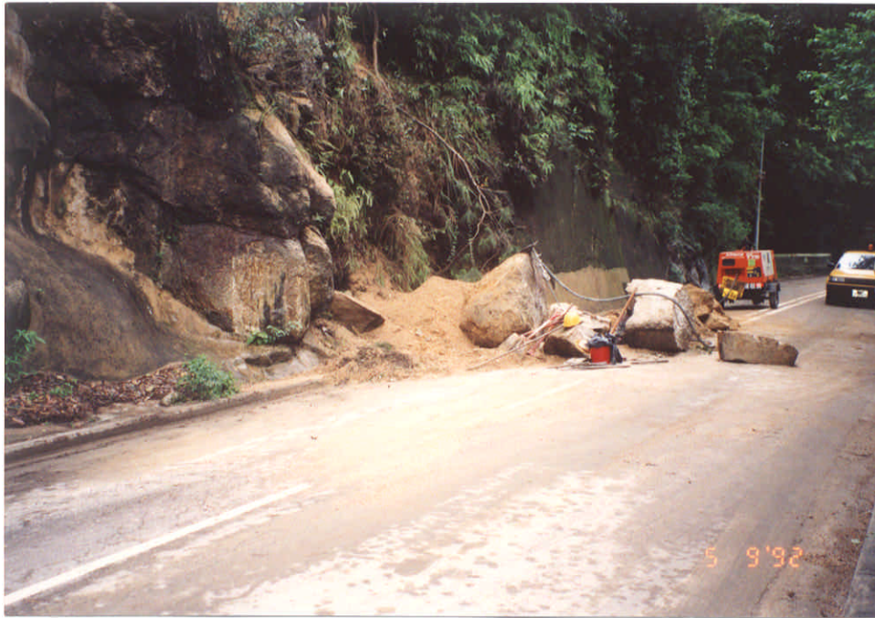
Negative No. I9224802 Taken on : 9-5-92 Description : Failure of a soil/rock cut slope resulting in the blockage of two road lanes.
