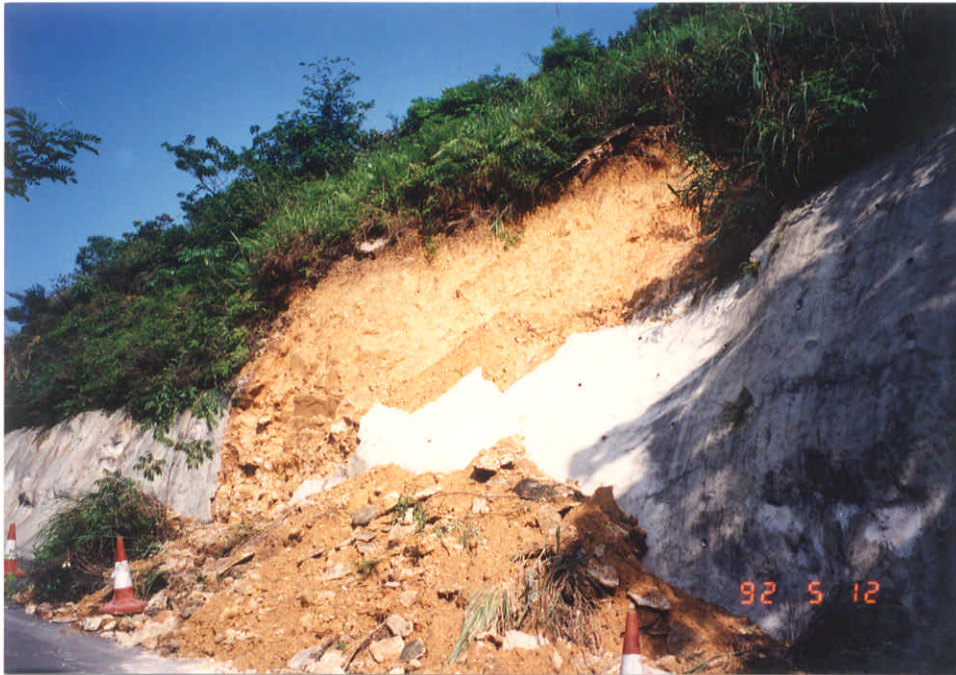
Negative No. MW9211521 Taken on : 12-5-92 Description : Failure of a soil cut slope resulting in the partial blockage of a road.
