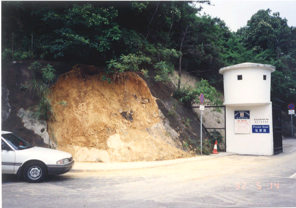
Negative No. I9224212A Taken on : 14-5-92 Description : Failure of a soil/rock cut slope affecting a pedestrian pavement.
