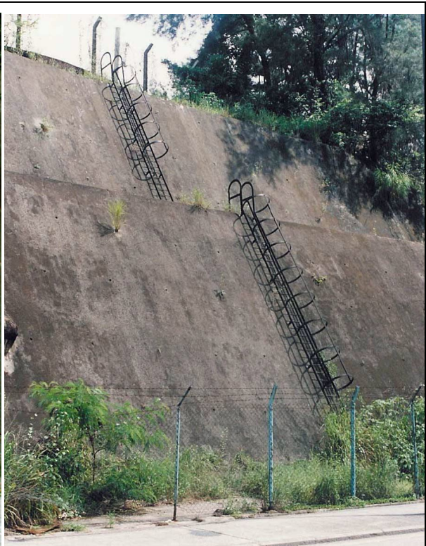
(b) Ladders with Safety Hoops
