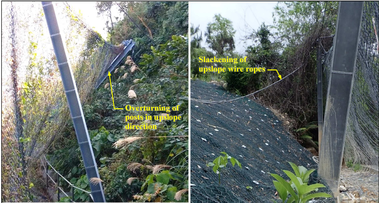
(a) Overturning of Posts
