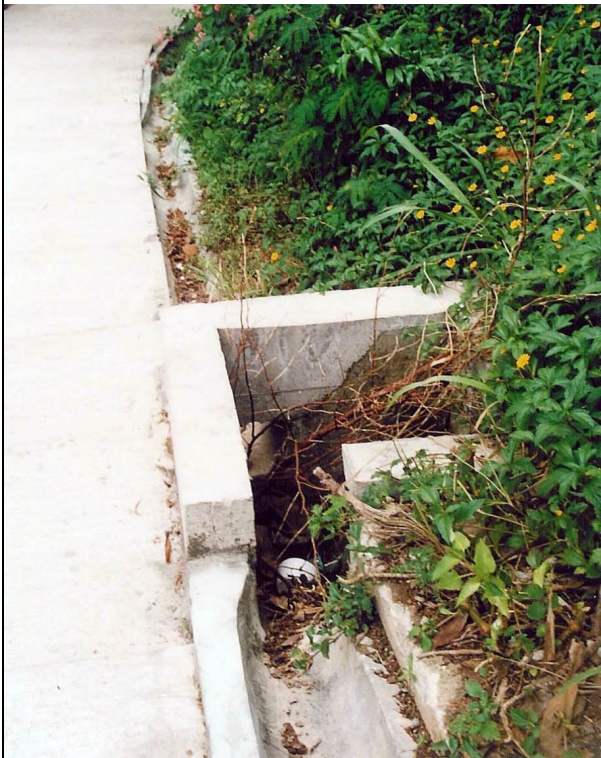
(c) Catchpit at Toe of Slope
