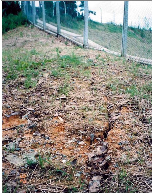
(a) Tension Crack on Slope
