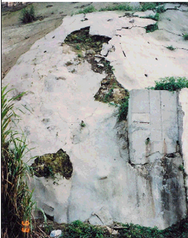
(c) Cracked Chunam Surface
