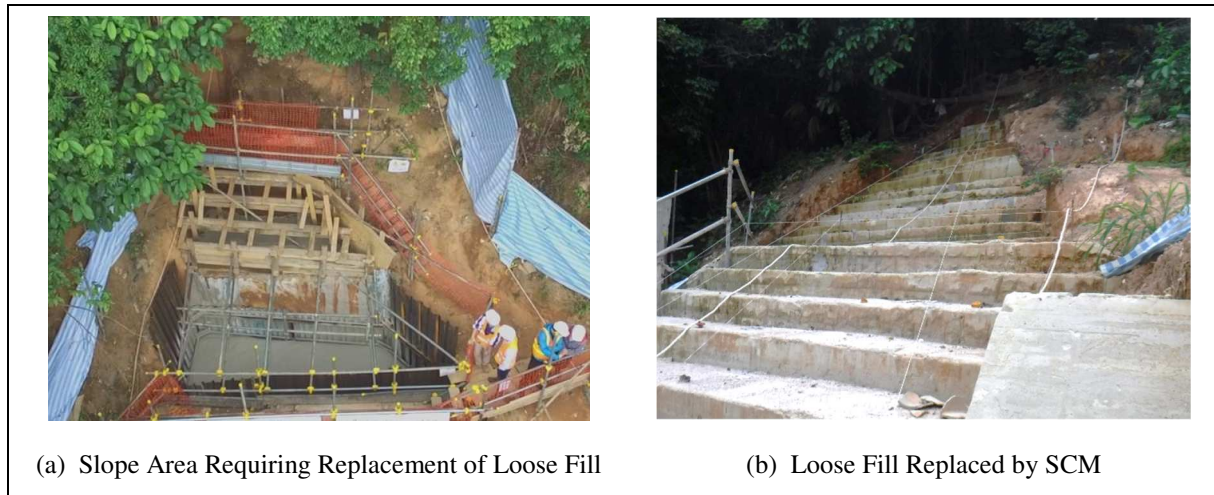
Figure 3.2 General Views of Slope Requiring Replacement of Loose Fill by Self-compacting Backfill Material
