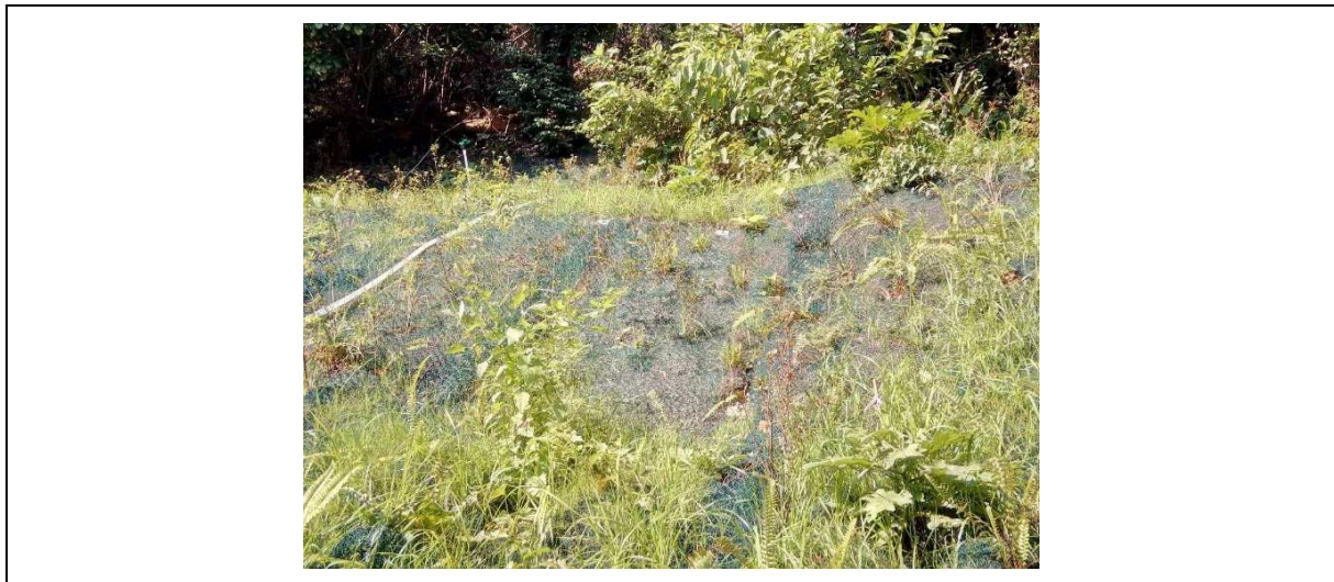
Figure 3.7 General View of Slope with Landslip Prevention and Mitigation Works involving Fill Replacement by Self-compacting Backfill Material Completed
