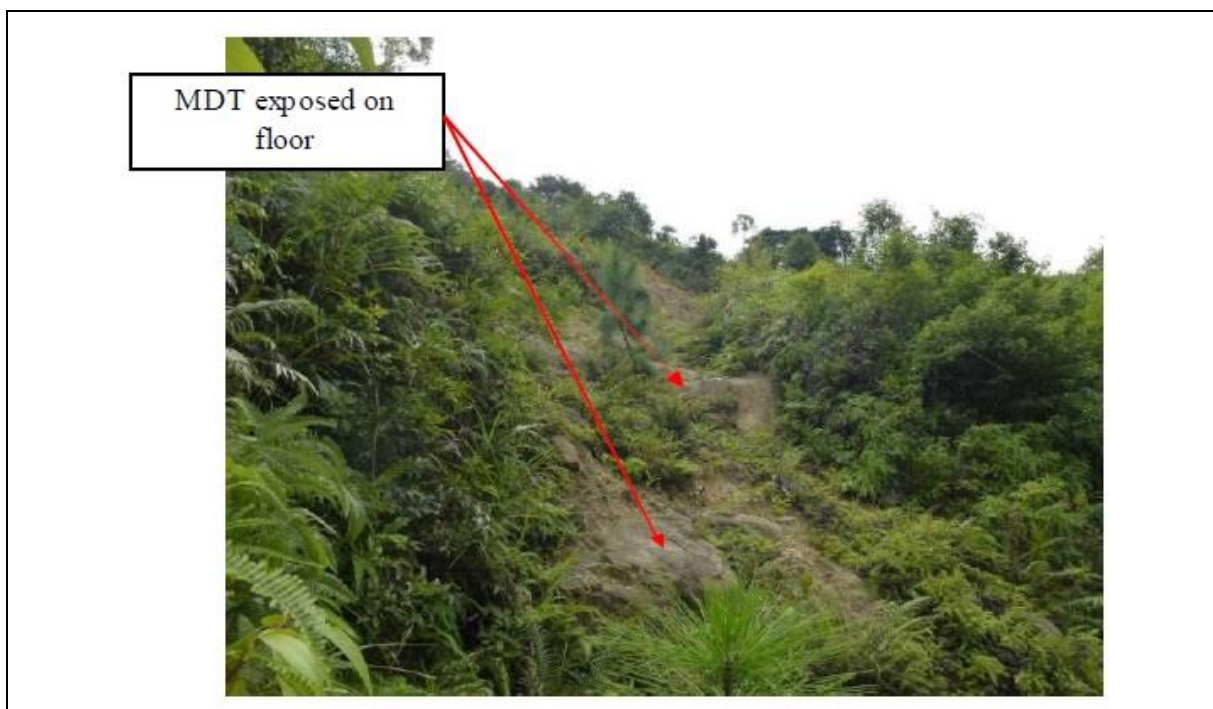
Plate D4.6 Exposed MDT at the Floor of Recent ENTLI No. 13NWB2703E (Landslide ID No. 80 in Catchment KSR56)
