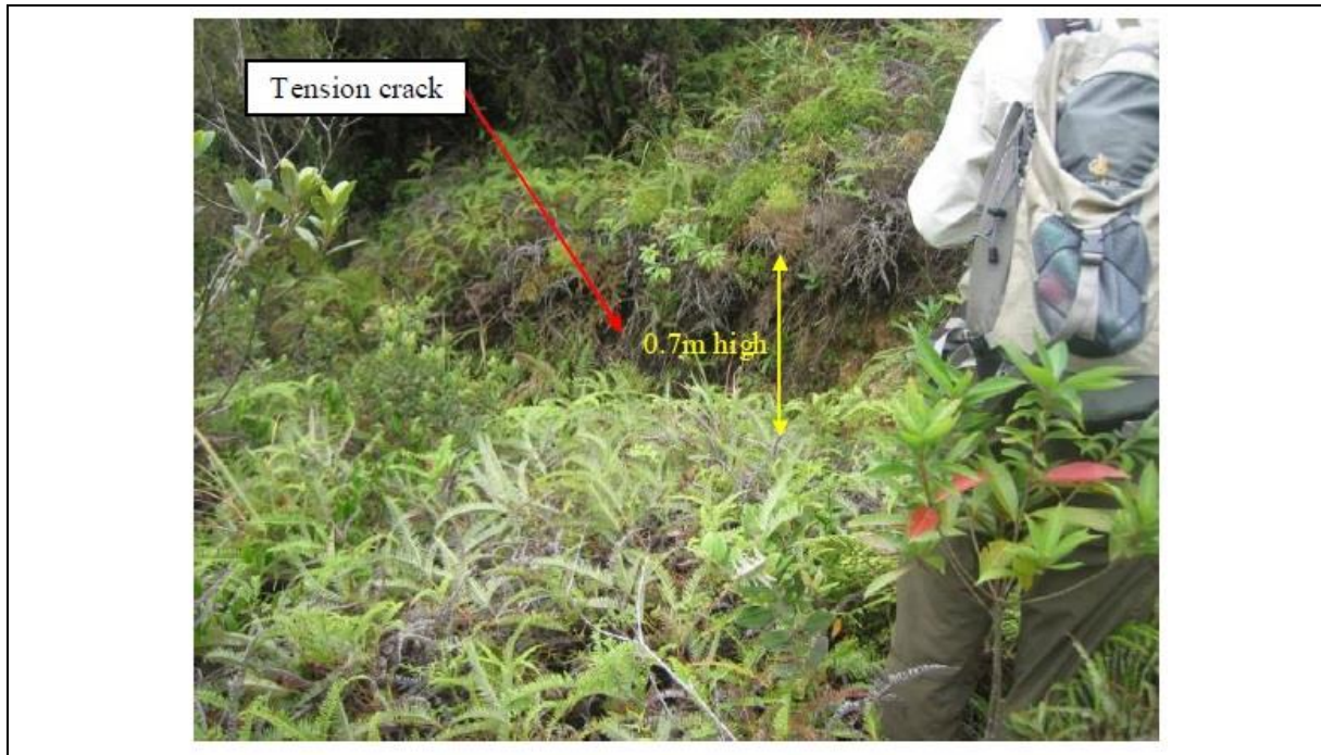
Plate D4.1 Tension Crack Extending towards the East Flank of Landslide ID No. 135 in Catchment 56A in this Study
