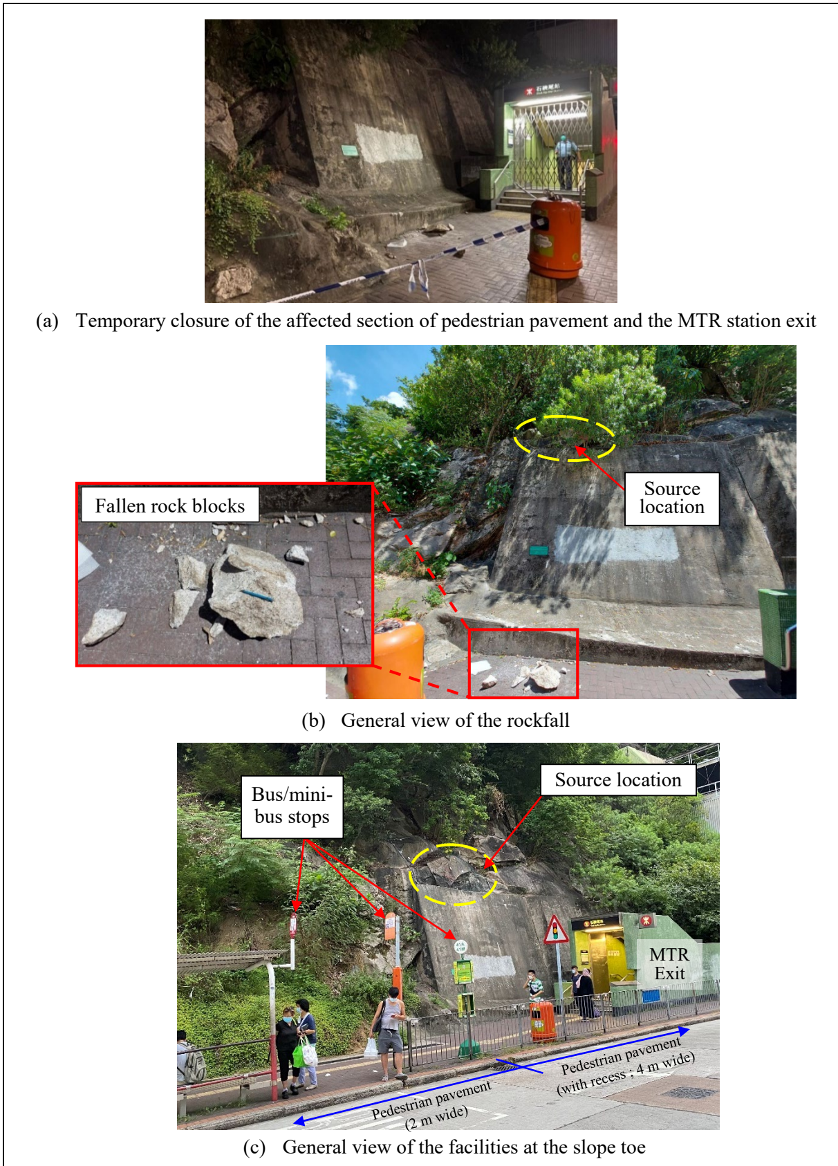
Figure 2.4 Views of the 15 July 2020 Rockfall at Woh Chai Street, Shek Kip Mei (Incident No. 2020/07/2723)
