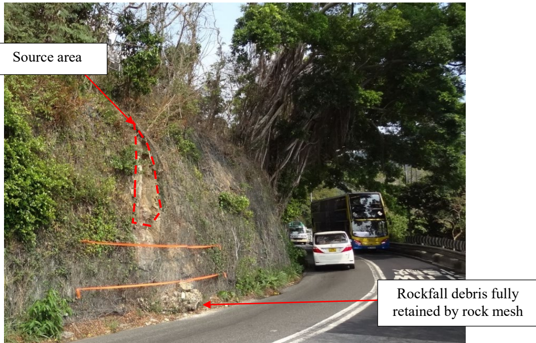
(a) Rockfall on a rock cut slope near the junction of Island Road and Repulse Bay Road in 2021
