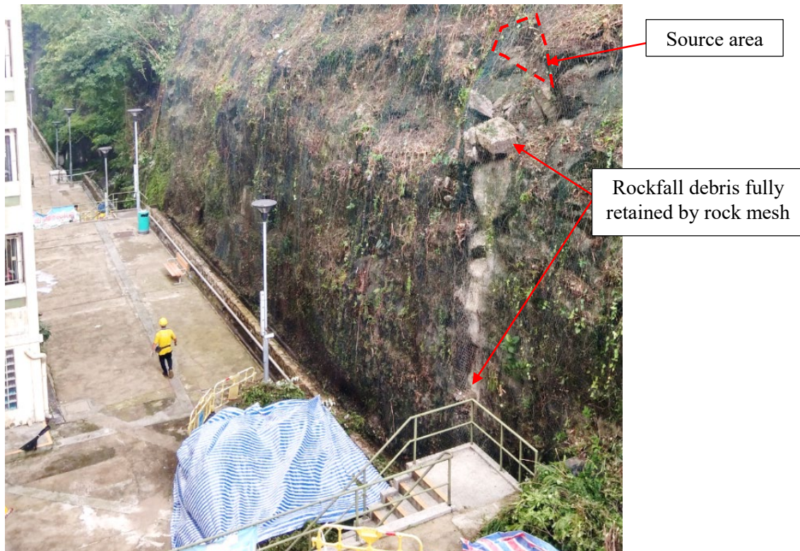
(b) Rockfall on a rock cut slope at No. 156 Kau Pui Lung Road, To Kwa Wan in 2021
