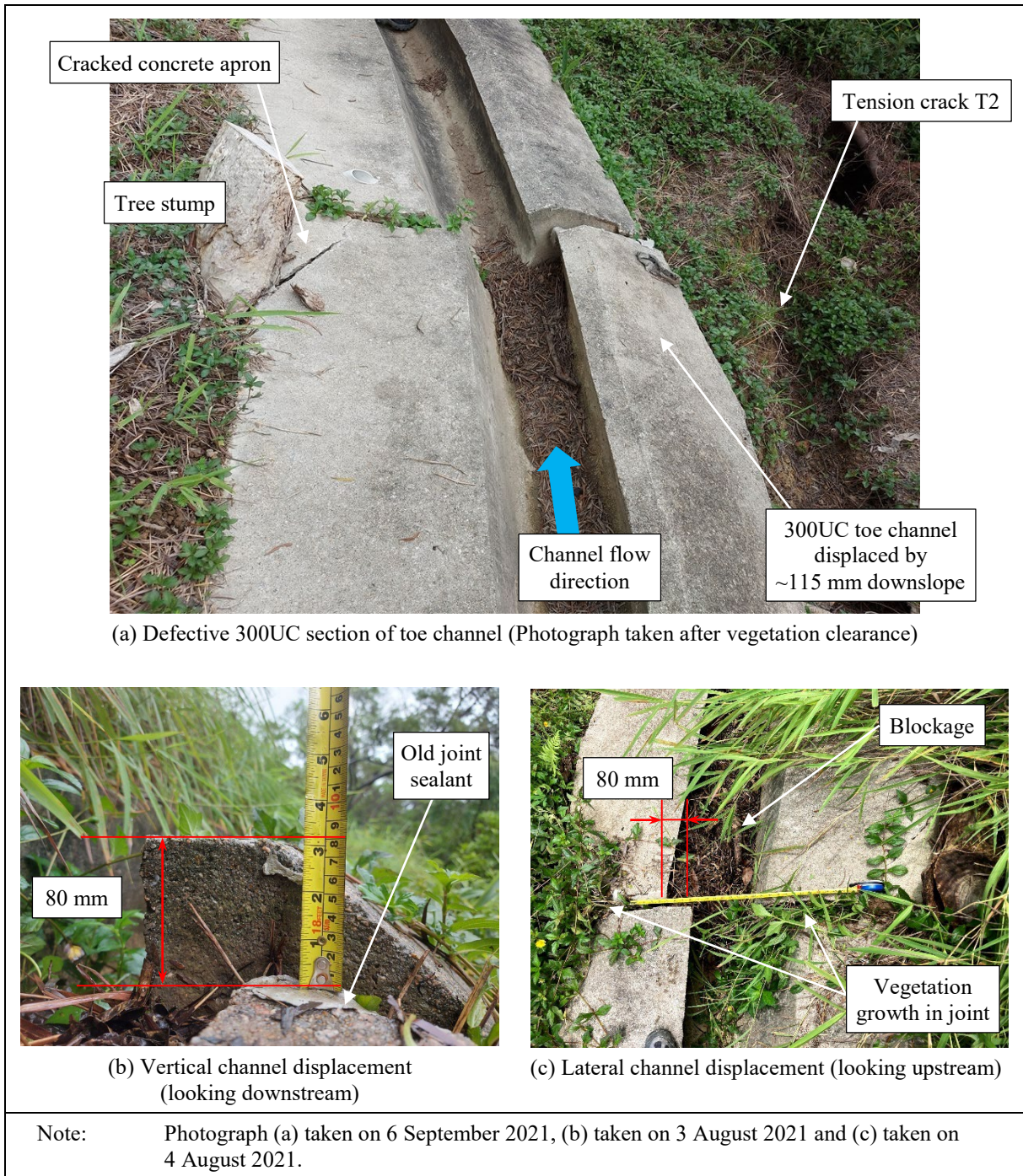
Figure 5.15 Defective 300UC Section (Photographs Taken on 3 August, 4 August and 6 September 2021)
