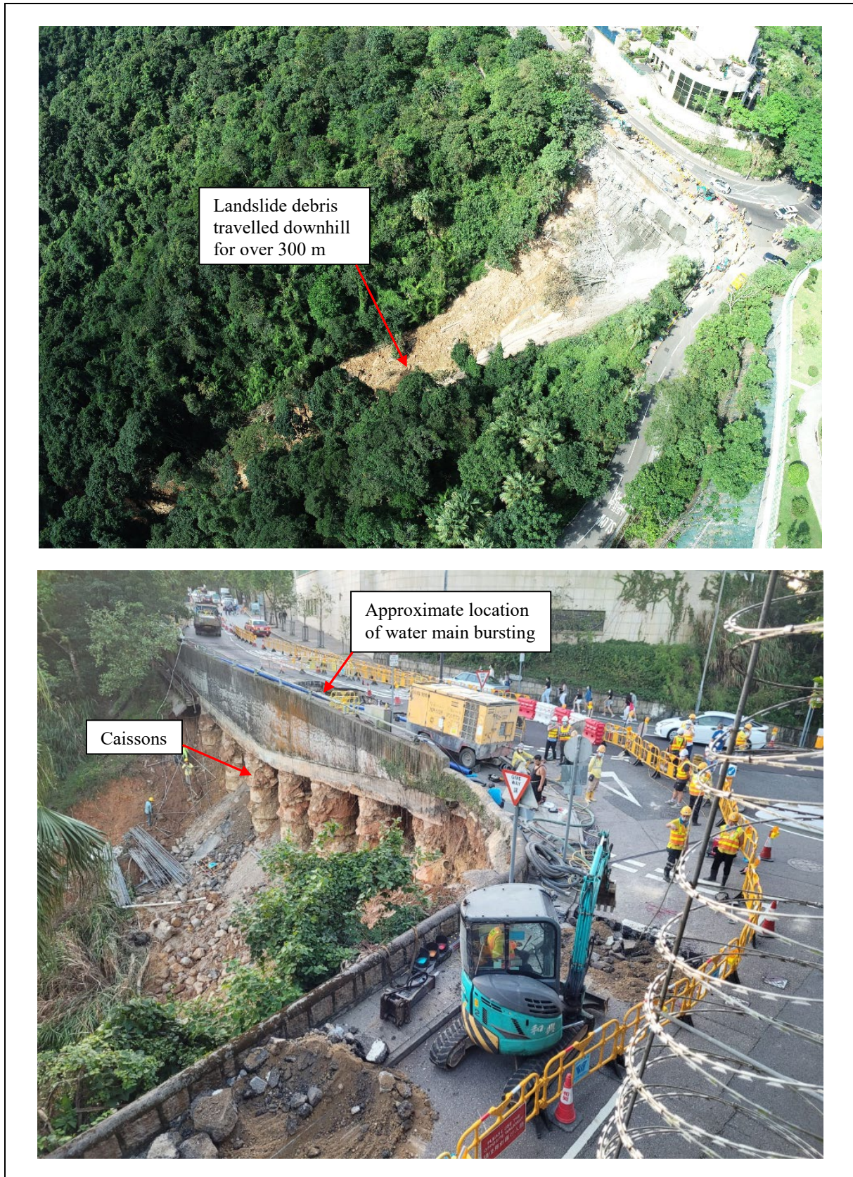
Figure B3 Flowslide at Peak Road (Incident No. 2021/11/3089)
