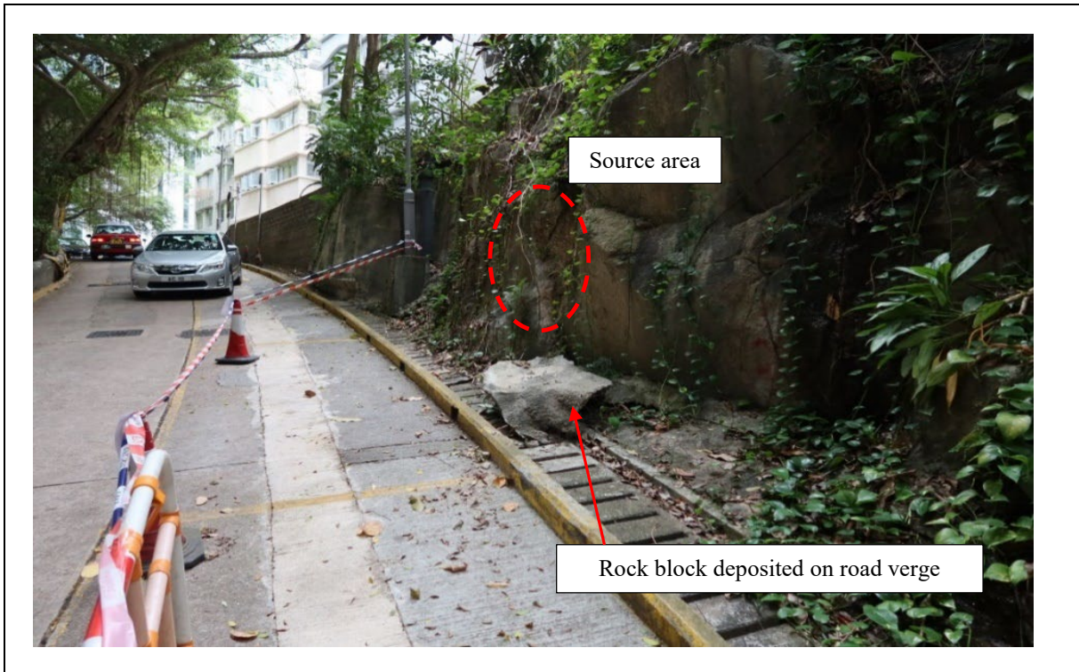
Figure B8 Rockfall in Happy Valley (Incident No. 2021/03/2868)
