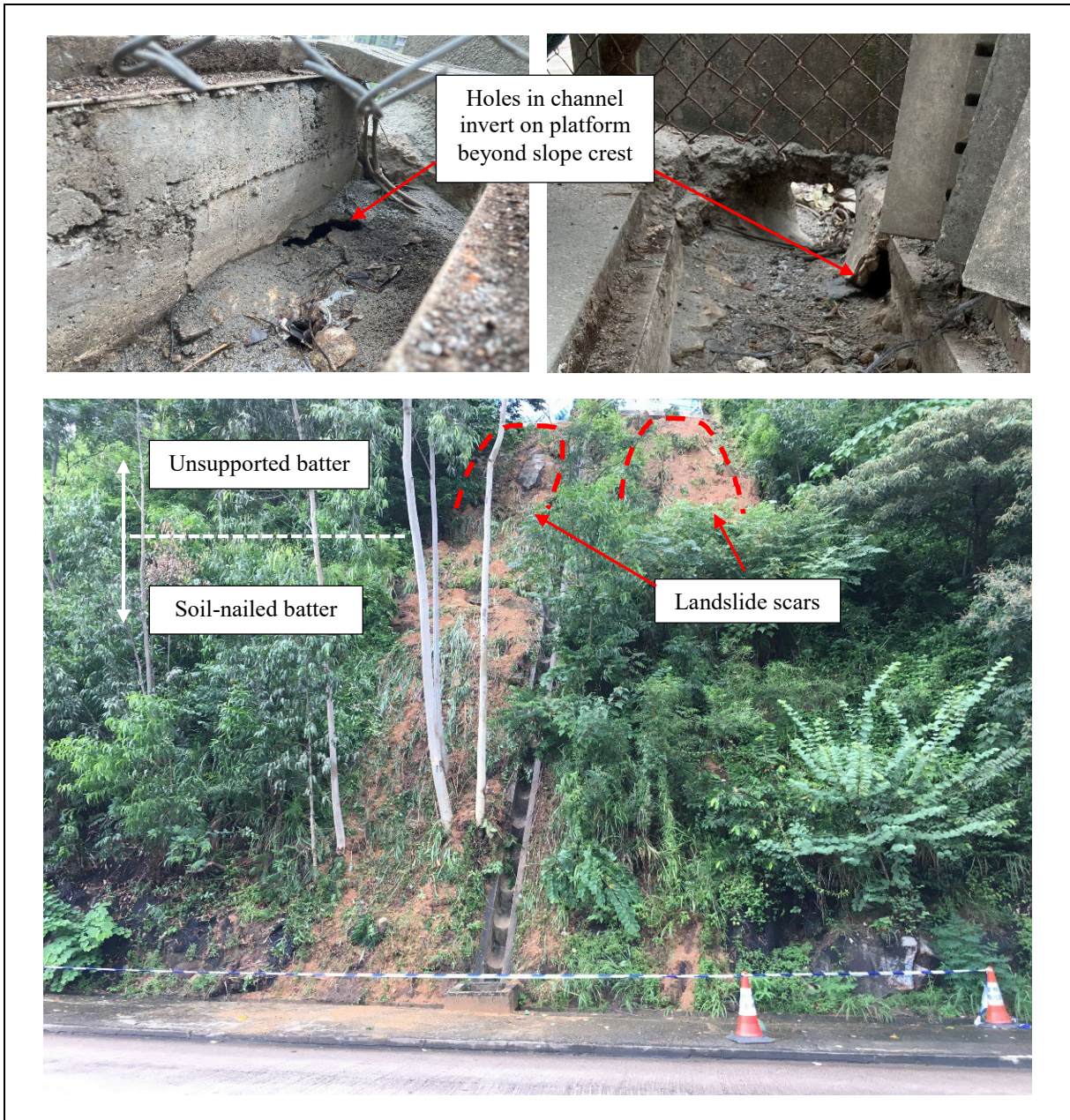
Figure B2 Sliding Failure at Castle Peak Road (Incident No. 2021/10/3045)
