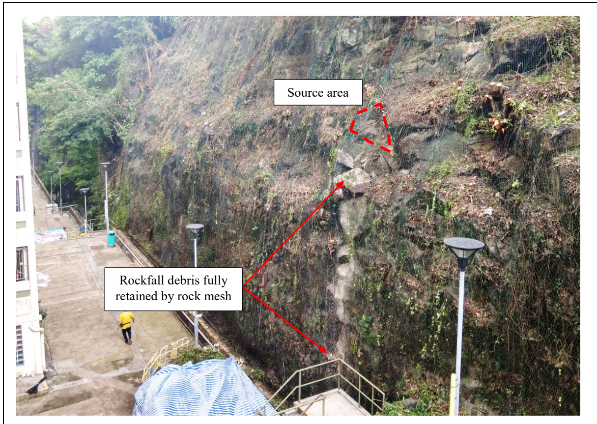
Figure B1 Rockfall in To Kwa Wan (Incident No. 2021/07/3005)
