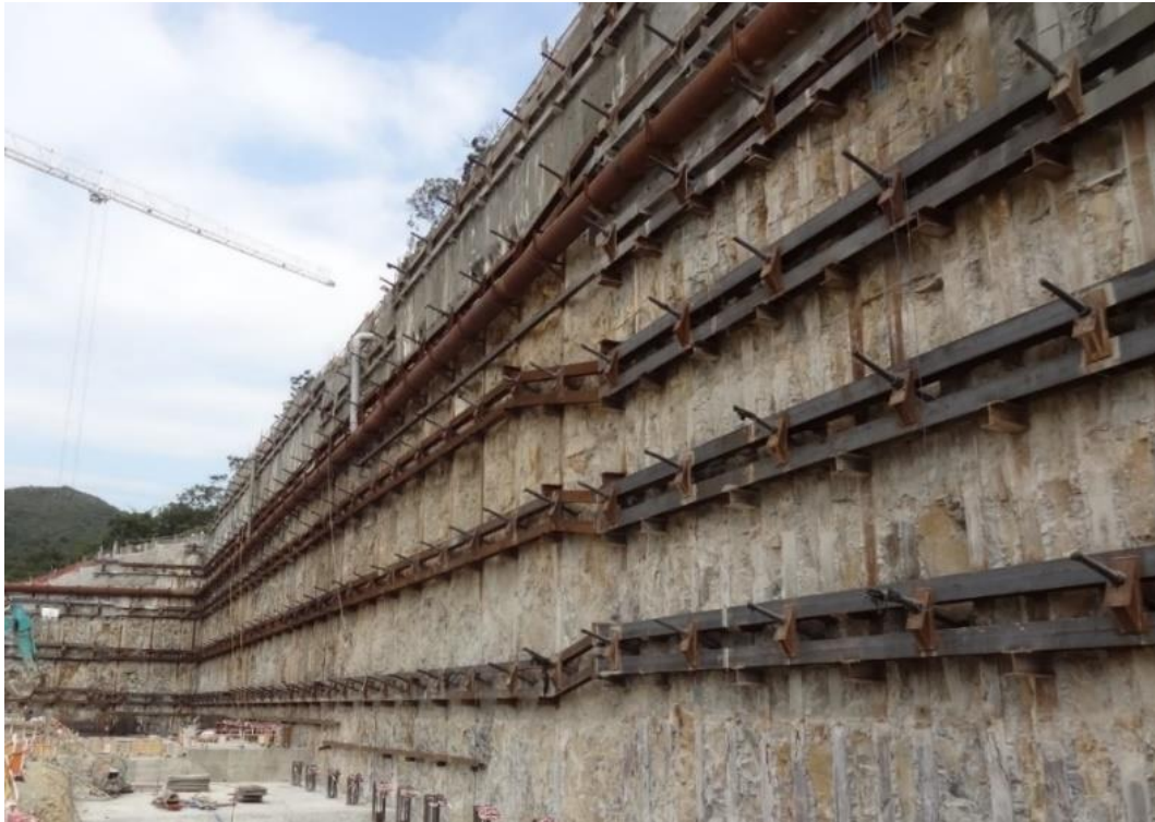
Figure 3.17 Retractable Prestressed Ground Anchor Support System at the Redevelopment of Grantham Hospital
