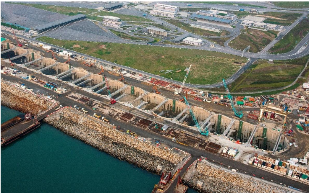
Figure 3.20 Multi-cell Circular Shaft for Cut-and-Cover Tunnel Construction under the Tuen Mun-Chek Lap Kok Link Project
