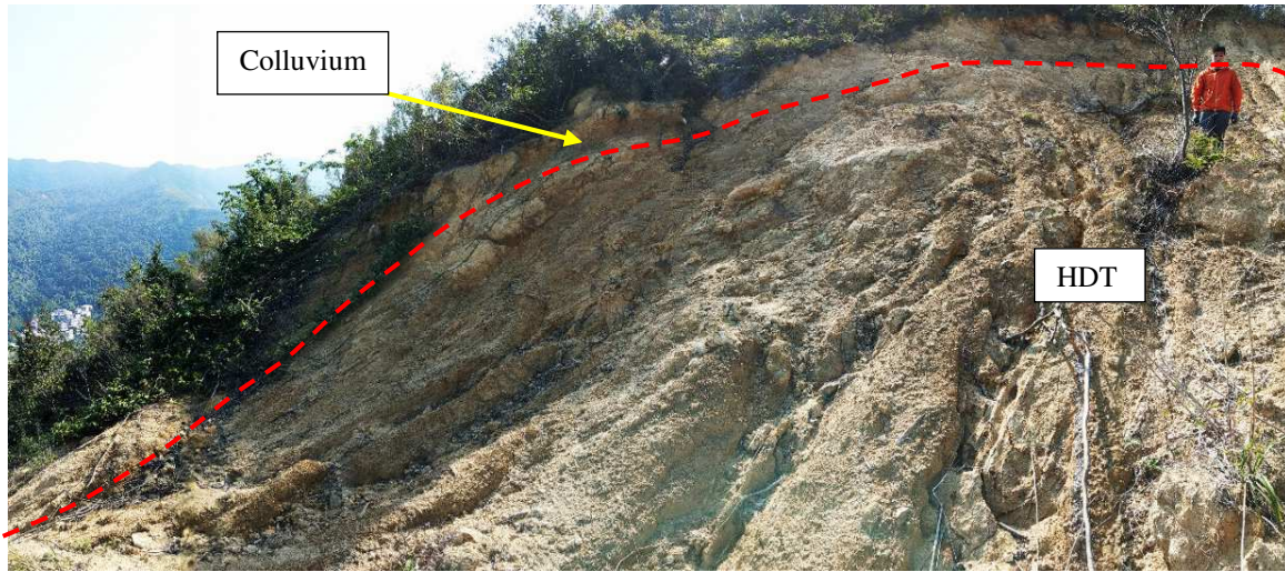
(b) View of L20 Showing Predominant Materials of the Landslides
