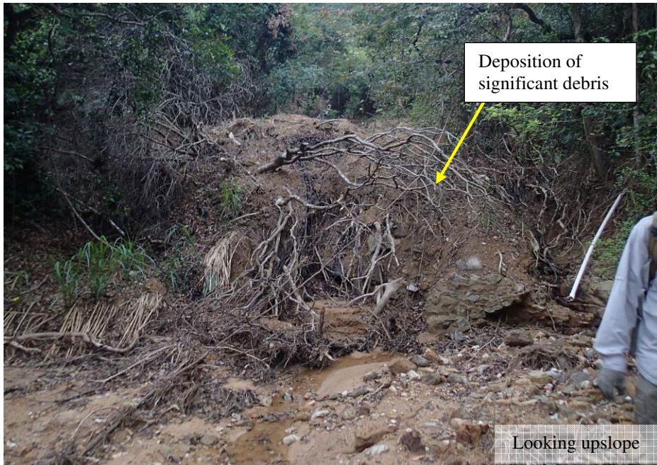
(e) View of Debris Trail from CH190 to CH200 Showing the Deposition Zone
