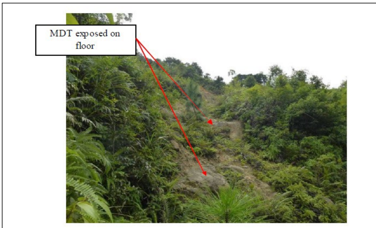
Plate D4.6 Exposed MDT at the Floor of Recent ENTLI No. 13NWB2703E (Landslide ID No. 80 in Catchment KSR56)
