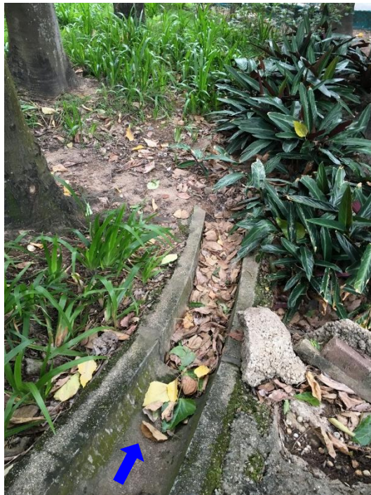
(c) Channel Blocked by Vegetation and Withered Leaves
