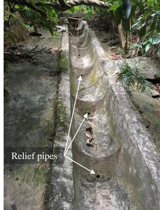
(t) Stepped Channel with Short Relief Pipes to Intercept Shallow Subsurface Flow
