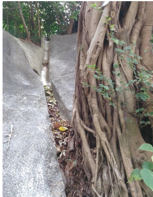
(h) Channel Blocked by the Root Growth of a Tree in Close Proximity
