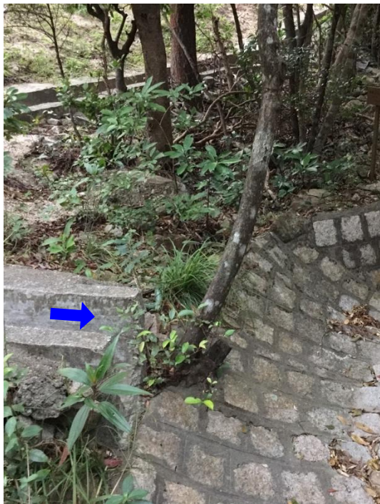
(k) Stone-Pitching below Discharge Point Enhancing the Resistance to Erosion
