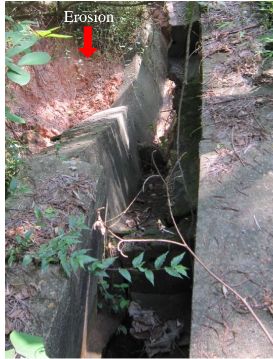
(b) Dislodged Channel Sidewall
