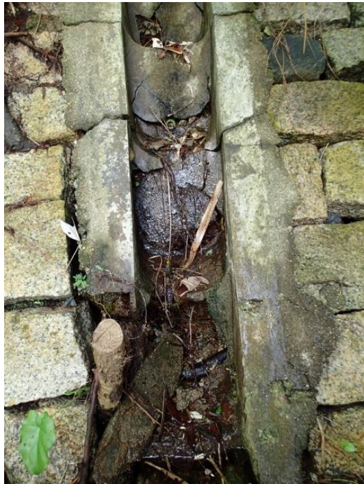
(a) Heavily Cracked Channel
