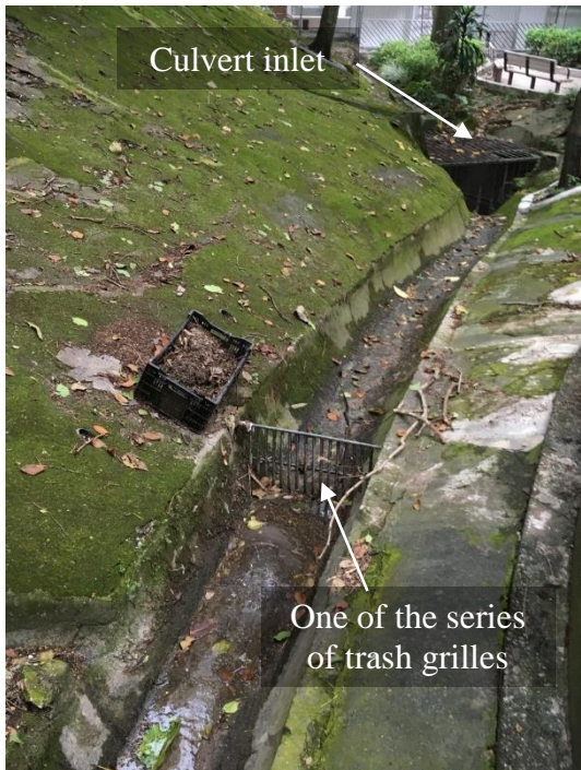
(o) Series of Trash Grilles at Upstream to Increase Solid Retention Capacity
