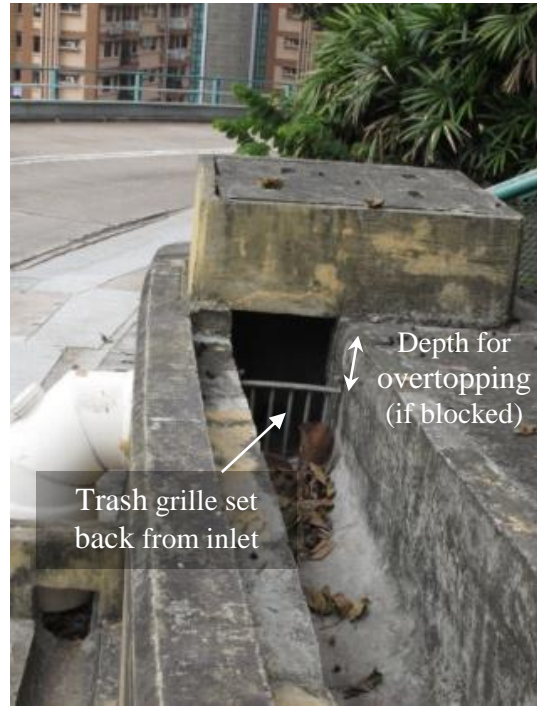
(n) Judiciously Located and Sized Trash Grille to Avoid Overflow in the Event of Blockage
