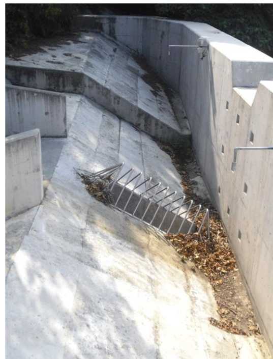
(p) Trash Rack on Slope Surface Reducing the Chance of Blockage
