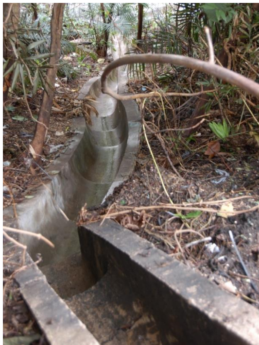
(c) Channel Section with Abrupt Change in Flow Direction being Prone to Spillage
