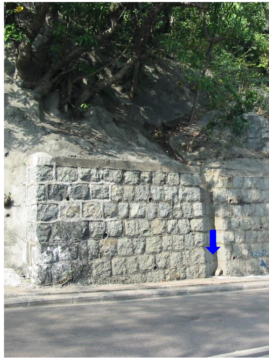
(b) Discharge of Runoff from Slope Directly onto Road Surface
