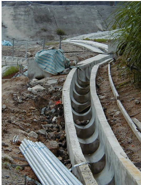
(e) Channel Sidewalls above Adjoining Ground with Erosion along the Side of Channel
