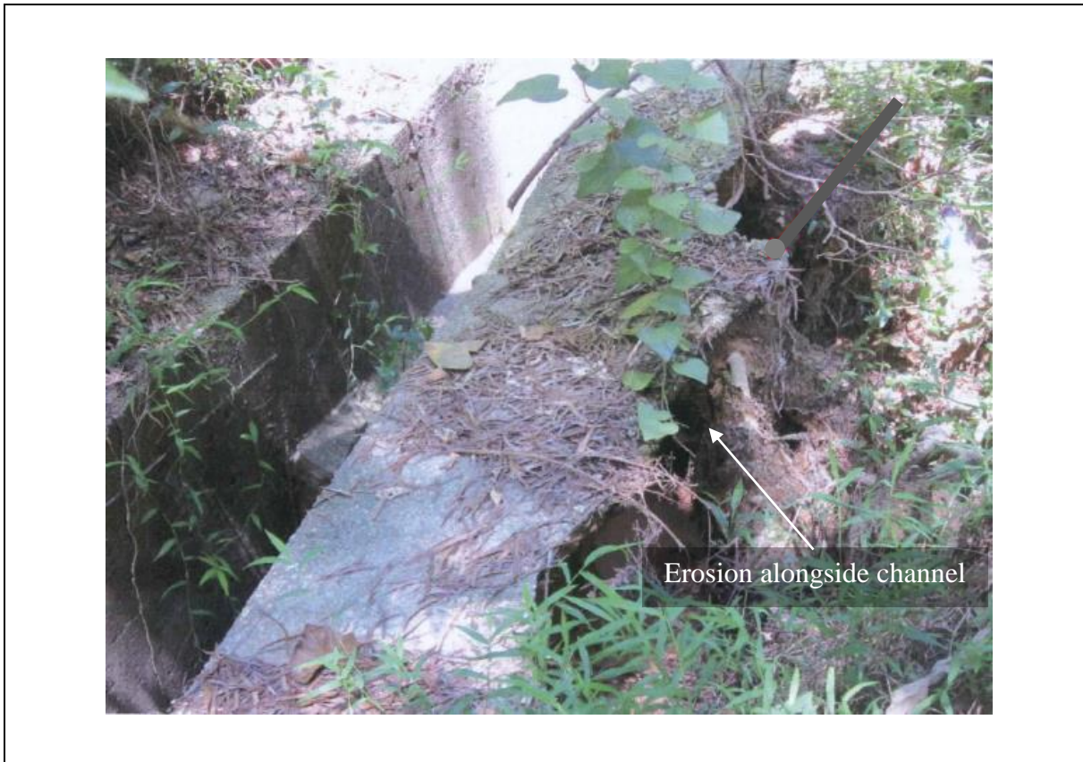
Figure 4.5 Example of Sign of Drainage Deficiency
