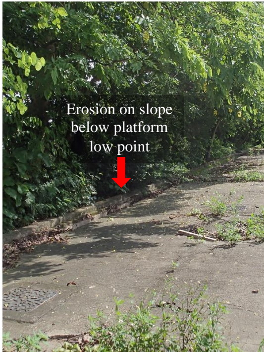
(a) Low Point with Insufficient Measure to Guard against Overflow
