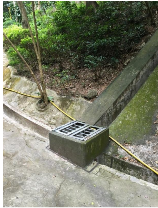
(f) Catchpit at Channel Junction for Flow Containment
