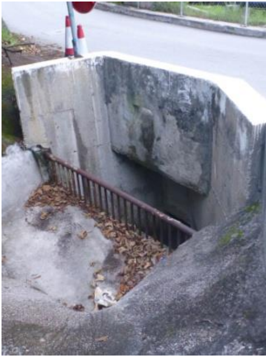
(q) Headwall at Drainage Inlet to Attenuate Peak Flow
