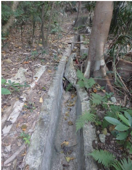
(g) Channel Damaged by the Root Growth of a Tree in Close Proximity
