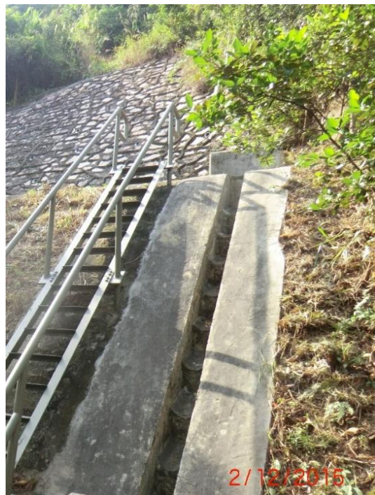
(l) Adequately Sized Channel Apron
