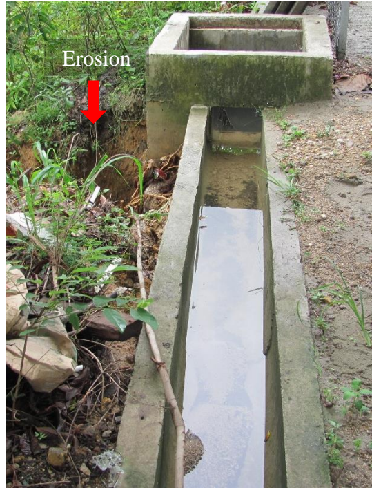
(d) Backing Up of Water within Blocked Channel and Catchpit
