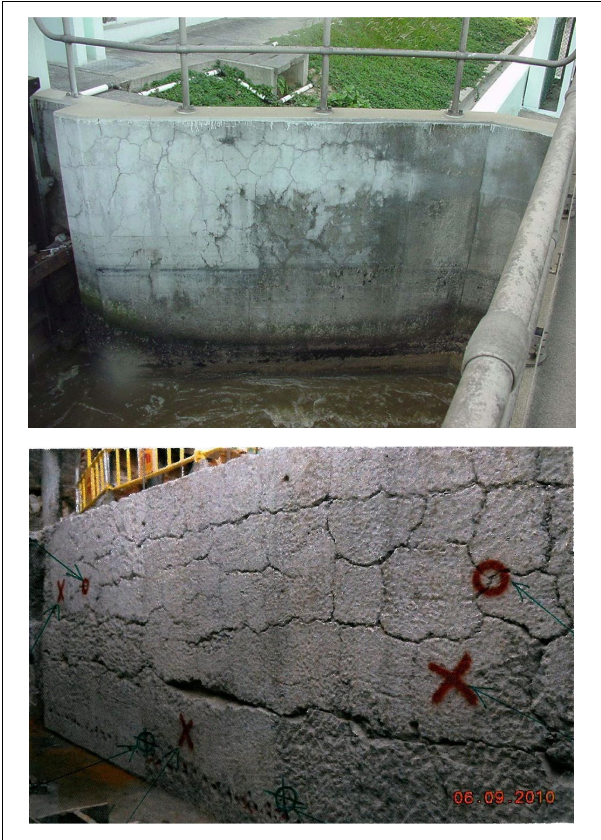
Figure 2.1 Typical Pattern of ASR Cracks
